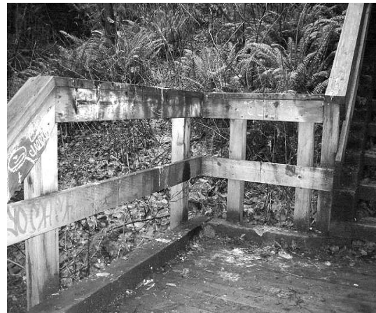
Stairs landing with burnt rails – after hours youth hangout?
